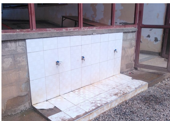
Figure 7: Public stand pipes with taps
