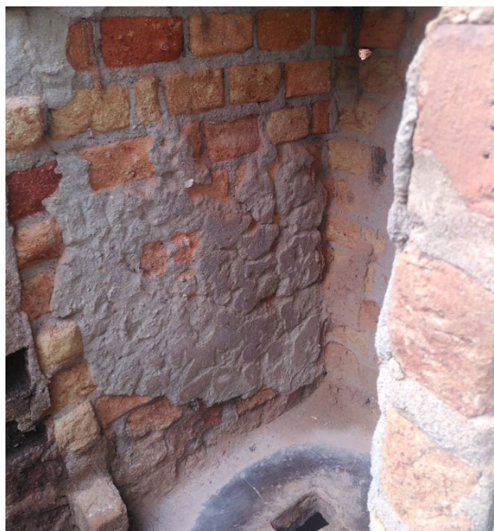
Figure 13: Unfinished pit latrine
