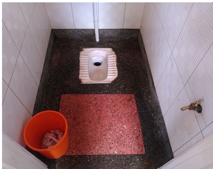
Figure 14: Very clean pit latrine
